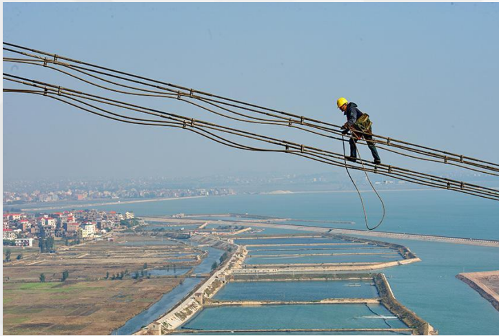
Walking on wire is dangerous
